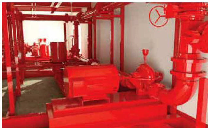
Interior Pump House Fire System
